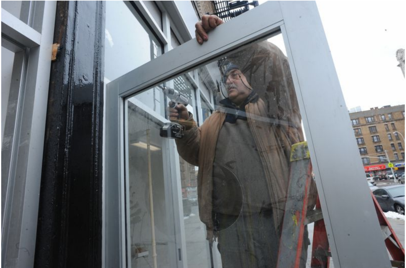
Alex Boyko installing door in ground floor storefront at 935 Kelly St. (Andrew Savulich/New York Daily News)
