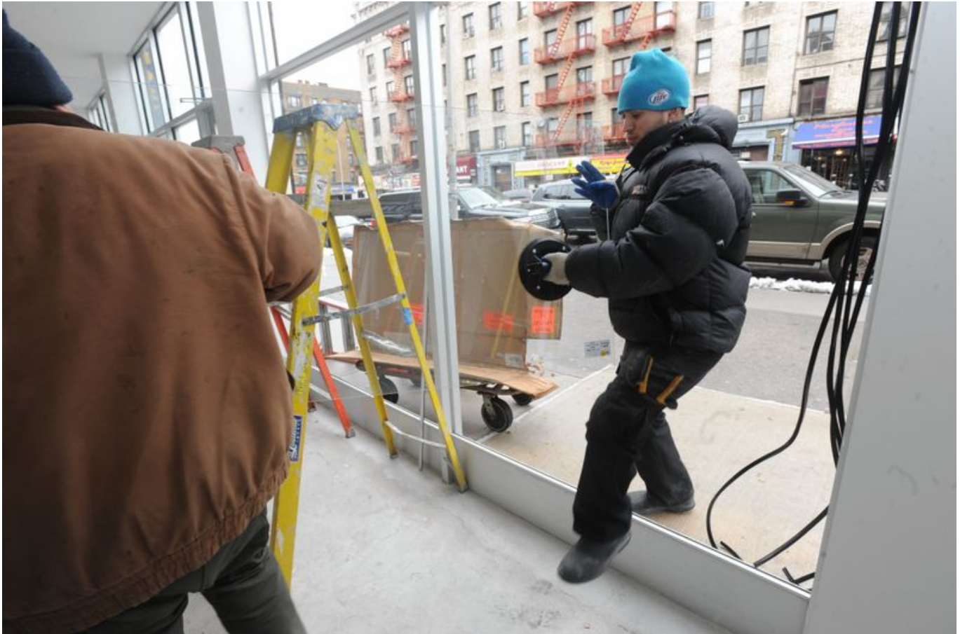
Workers installing windows in ground floor storefront at 935 Kelly St. (Andrew Savulich/New York Daily News)
